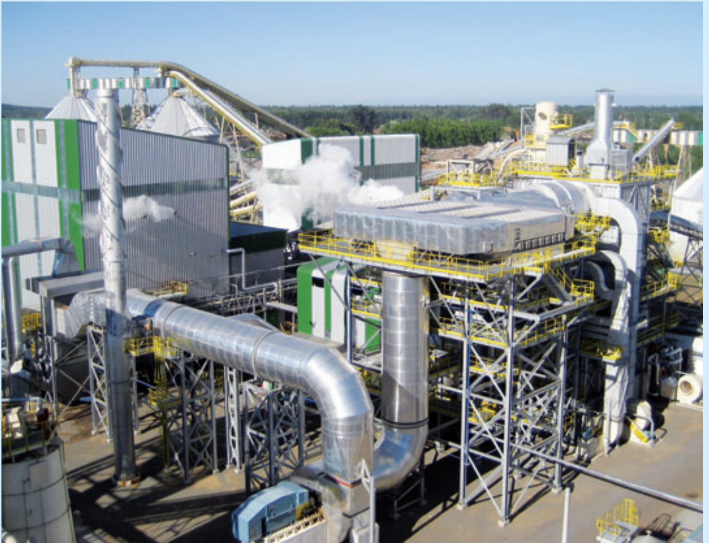
SES energy plant in Chile
