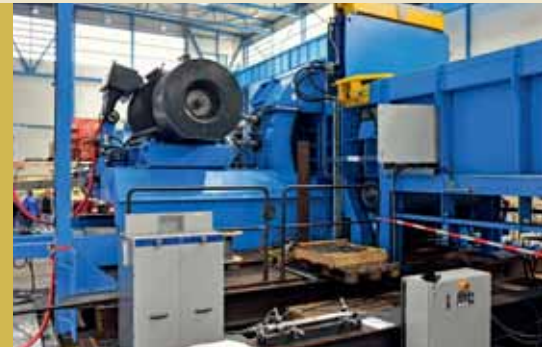
Main drive motor
