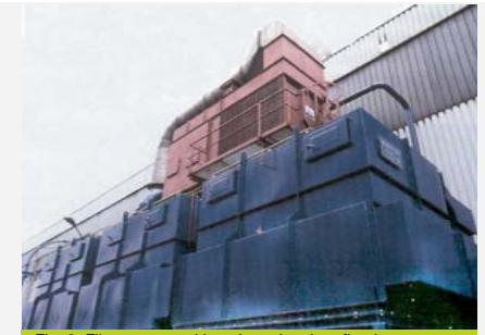
Fig. 3: Filter system with activated carbon fixed bed adsorber
