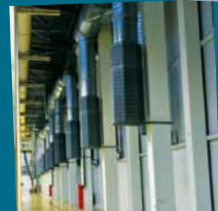
Fresh air supply for the hall
