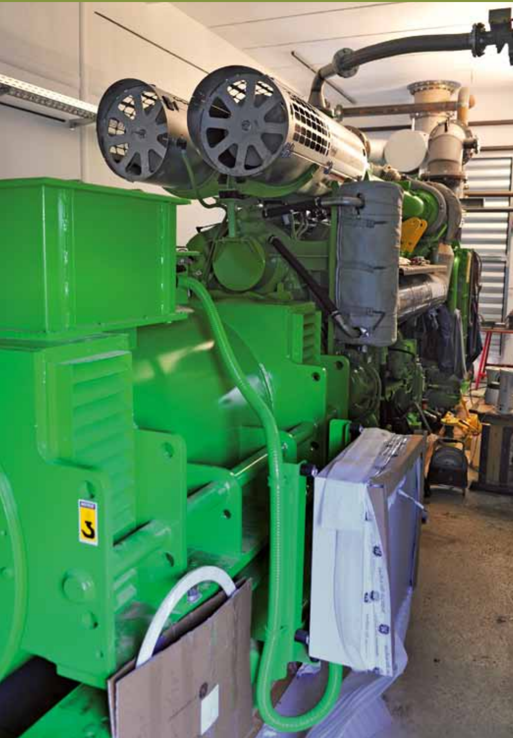
Generator with motor
