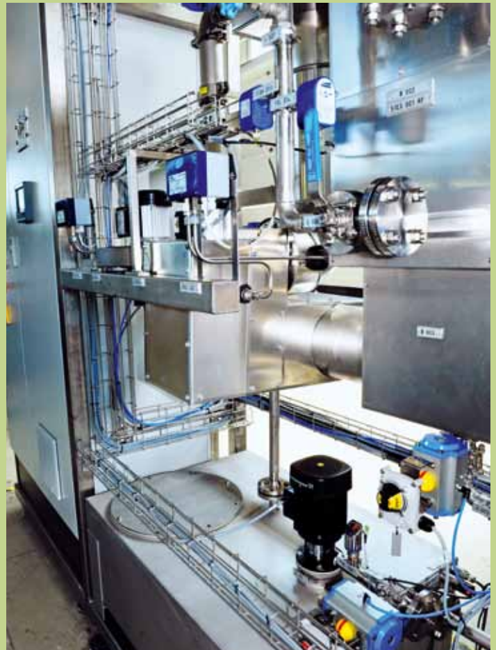
Left: vacuum system of the drying plant, right: cold water system for condensate separation
