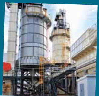
Silo for surface layer and core layer particles
