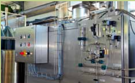
Two-drum drying plant: left side – control panel of the drying chamber door and drum conveyor, right side – switchgear of the fire-extinguishing system
