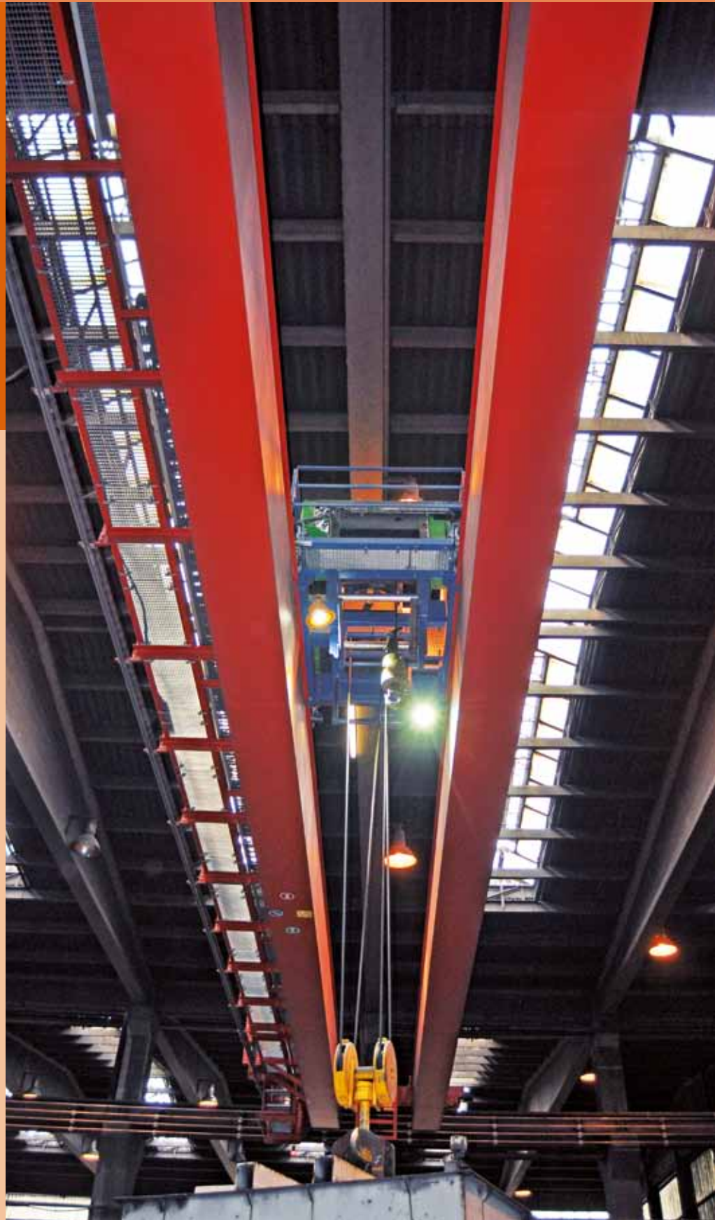
SGL Group, Meitingen, ring kiln area: SKT double girder bridge crane with view to the crab trolleys and load pick-up
