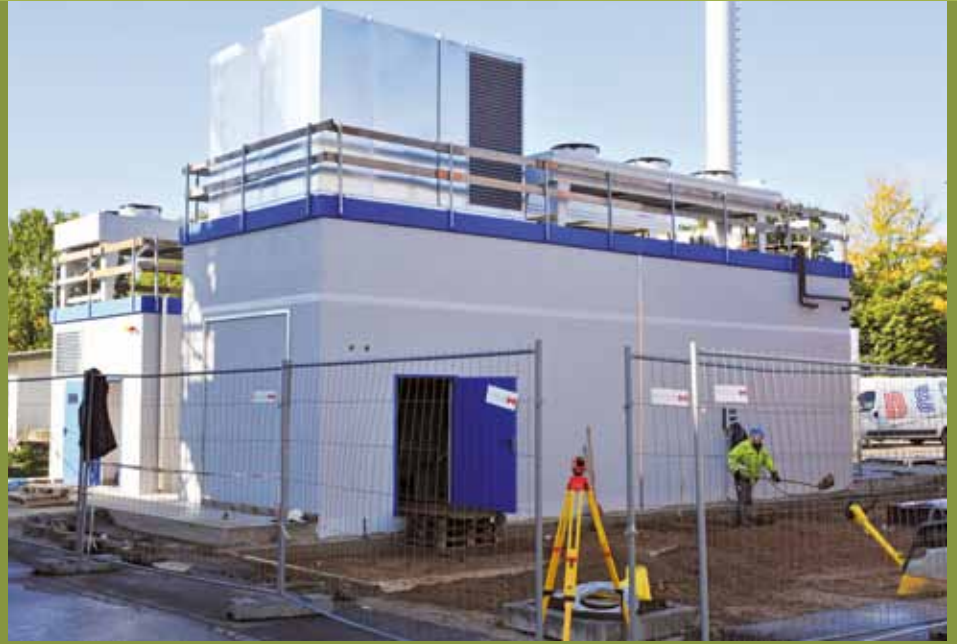
Combined heat and power unit
