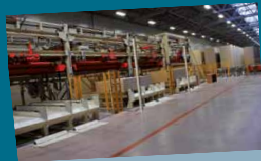
Stacking boxes with unfinished board storage for the feeding of the short-cycle press
