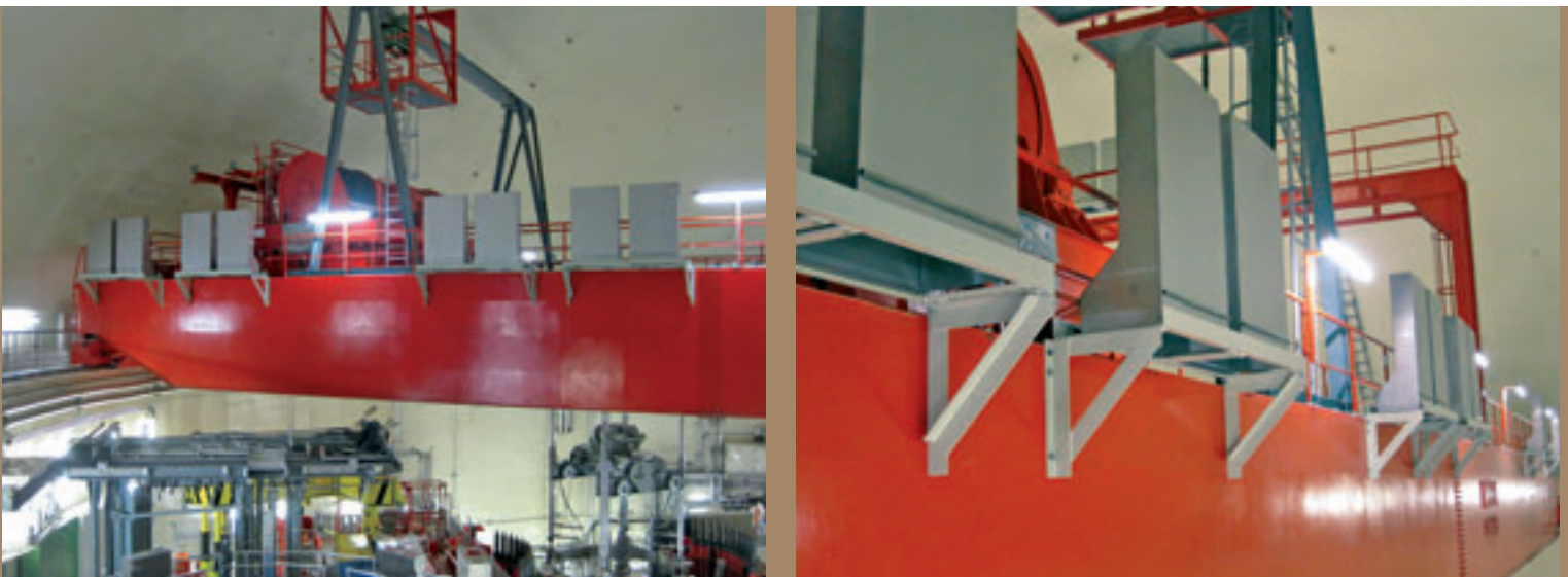
Operation of the hydrogen recombining system at a polar crane in the nuclear power plant
