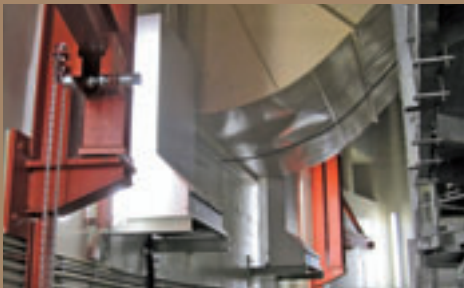
Different locations of use (from top to bottom): on the steam generator, in the controls and instruments room, inside pipe channels
