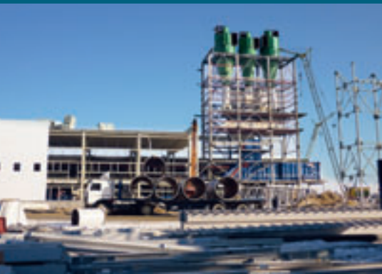
Matformer bunker for resinated fibers
