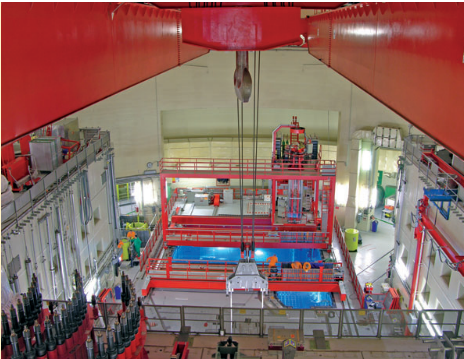
The polar crane in the foreground with view of the refueling machine
