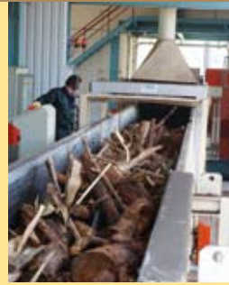
Wood feed to the chipper
