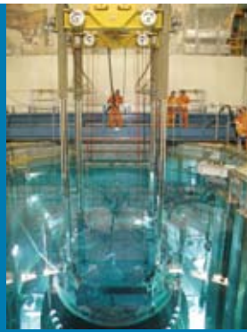
Transport of the sealing lid with the SNT lifting device inside the containment
