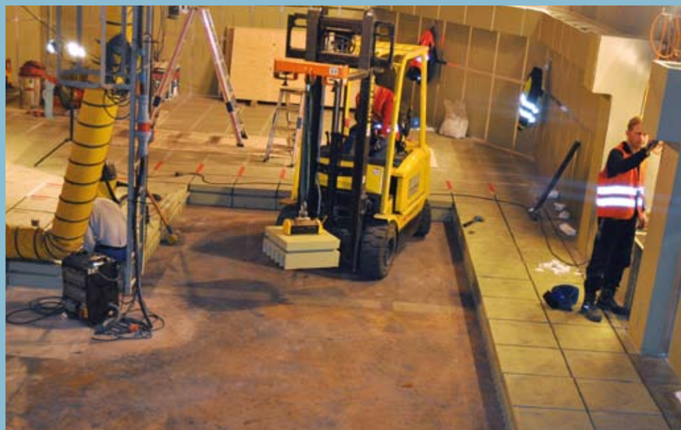
Logistical masterstroke – the transport of elements weighing up to 800 kg (0.9 US tons) in a tight space
