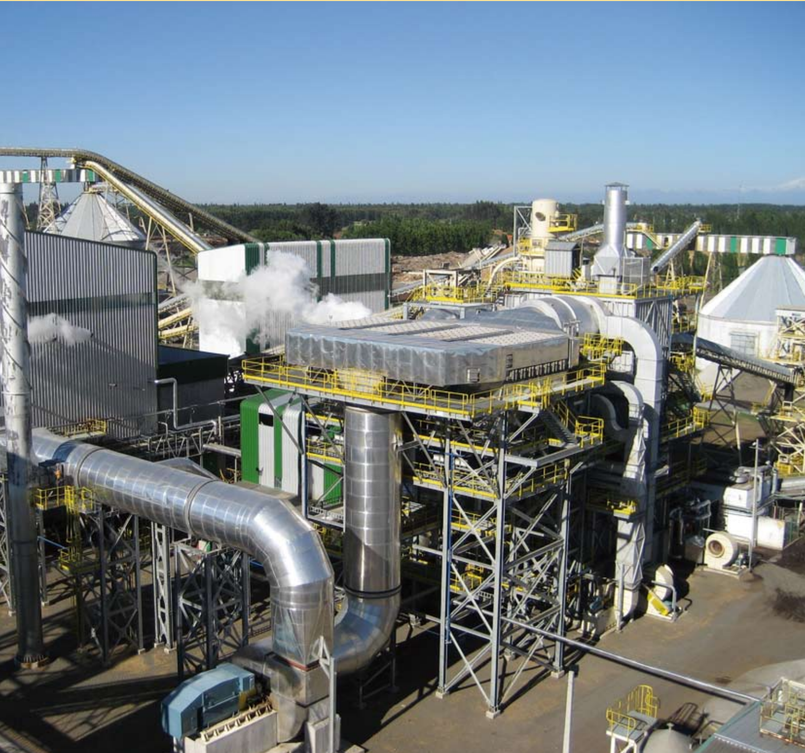
Energy plant SES Chile
