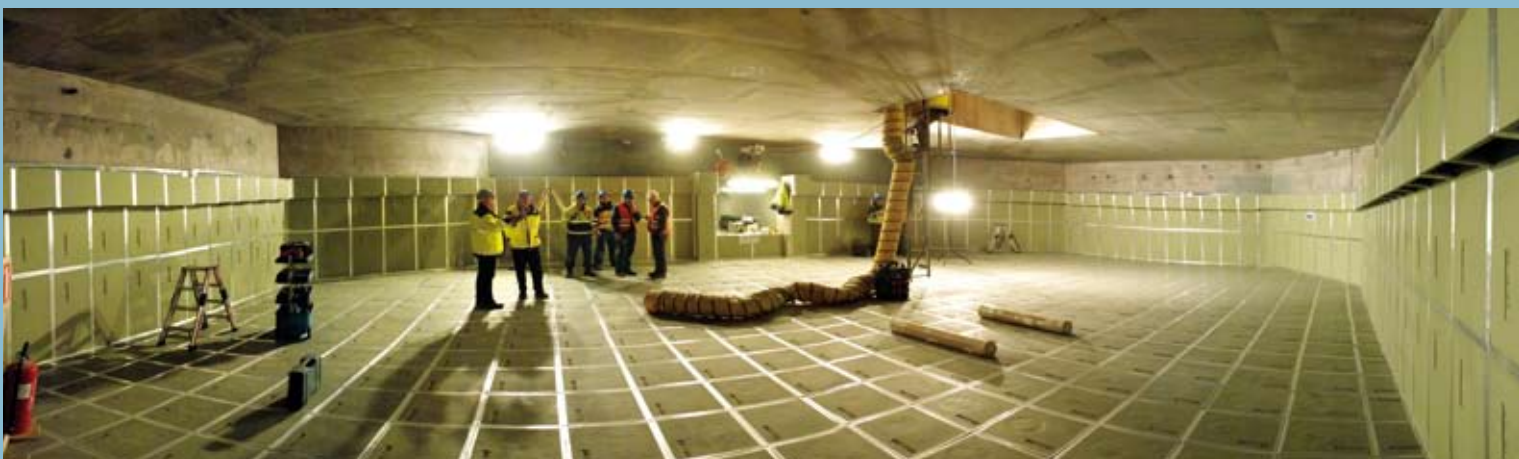
The spreading room with the installed cooling structure of the Core Catcher
